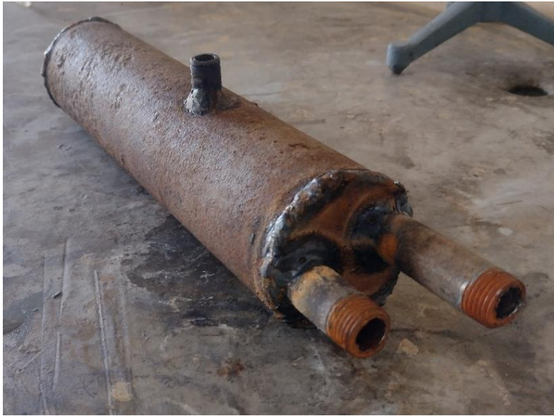
Figure 15: Manifold Outlets View (Source: Own Work)
